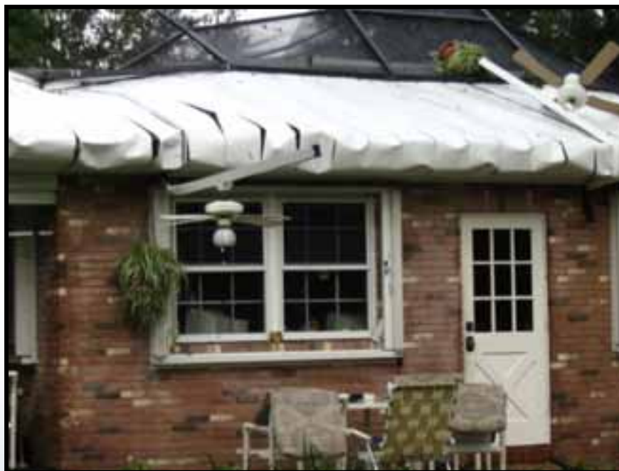
Tornado damage in Brandon, FL
